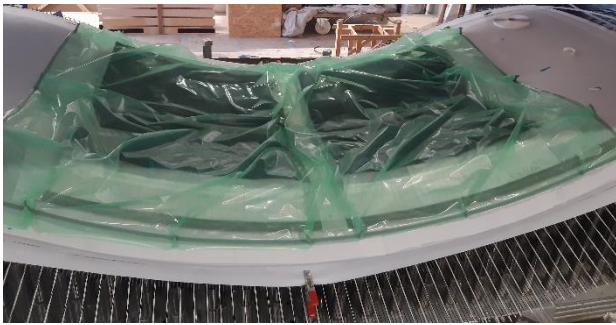
a: Preparation of the vacuum infusion of two sandwich panels on the adaptive mould
